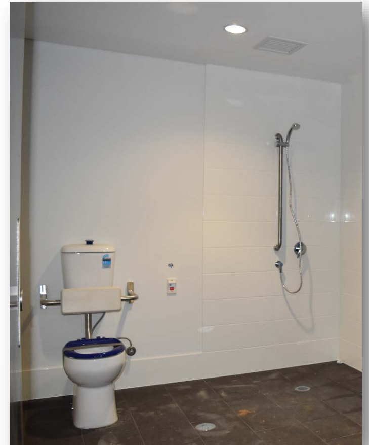
Toilet and Shower in the Gymnasium at the new Sports, Recreation and Community Complex
